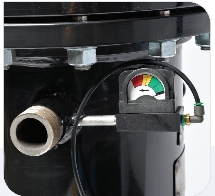
Differential pressure gauge (DPG) mounted and piped for ease of trouble shooting.
